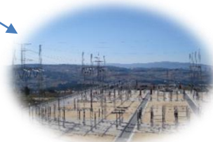
400/220 kV Armamar substation
