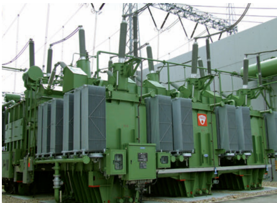
Auto-transformer at the substation of Pedralva
