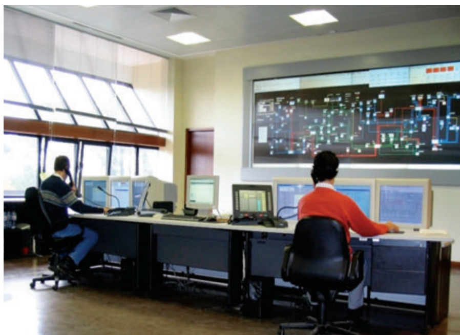
National Grid Control Centre
